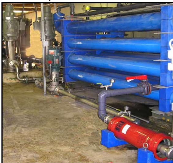
Right to left: PX-220B, RO Rack, Booster Pump and HP Pumps
